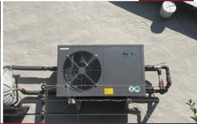
Installed heat pump
