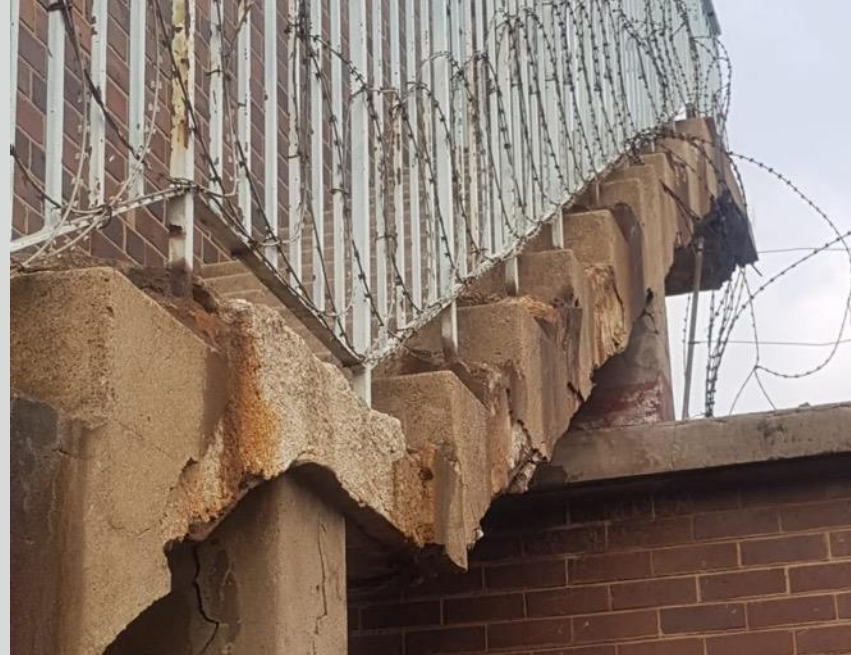
Before - Damaged unsafe stairways
