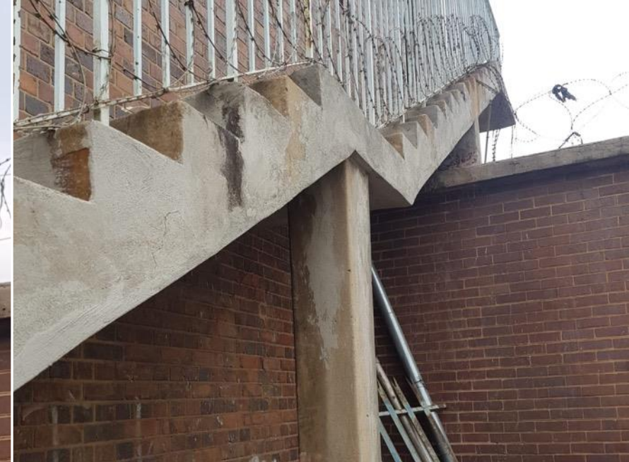
After – stairways meets the safety requirements
